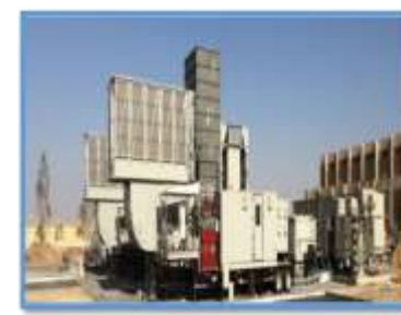
Mobile Units (40 x 25MW )Total 500 MW Distributed in Upper Egypt
